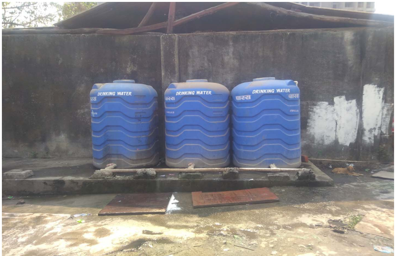
DRINKING WATER FACILITY AT SITE FOR LABORS
