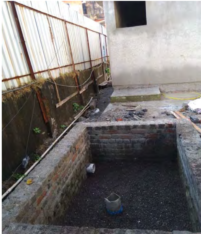
RAIN WATER HARVESTING SYSTEM
